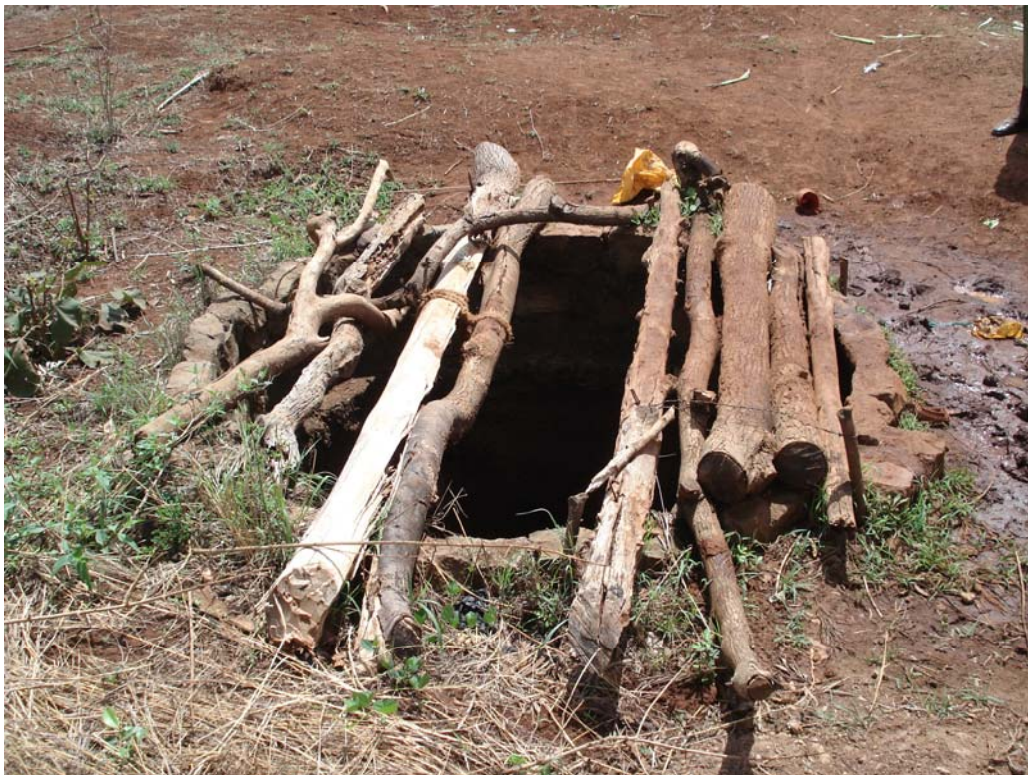
Plate 14: Improperly covered water well
