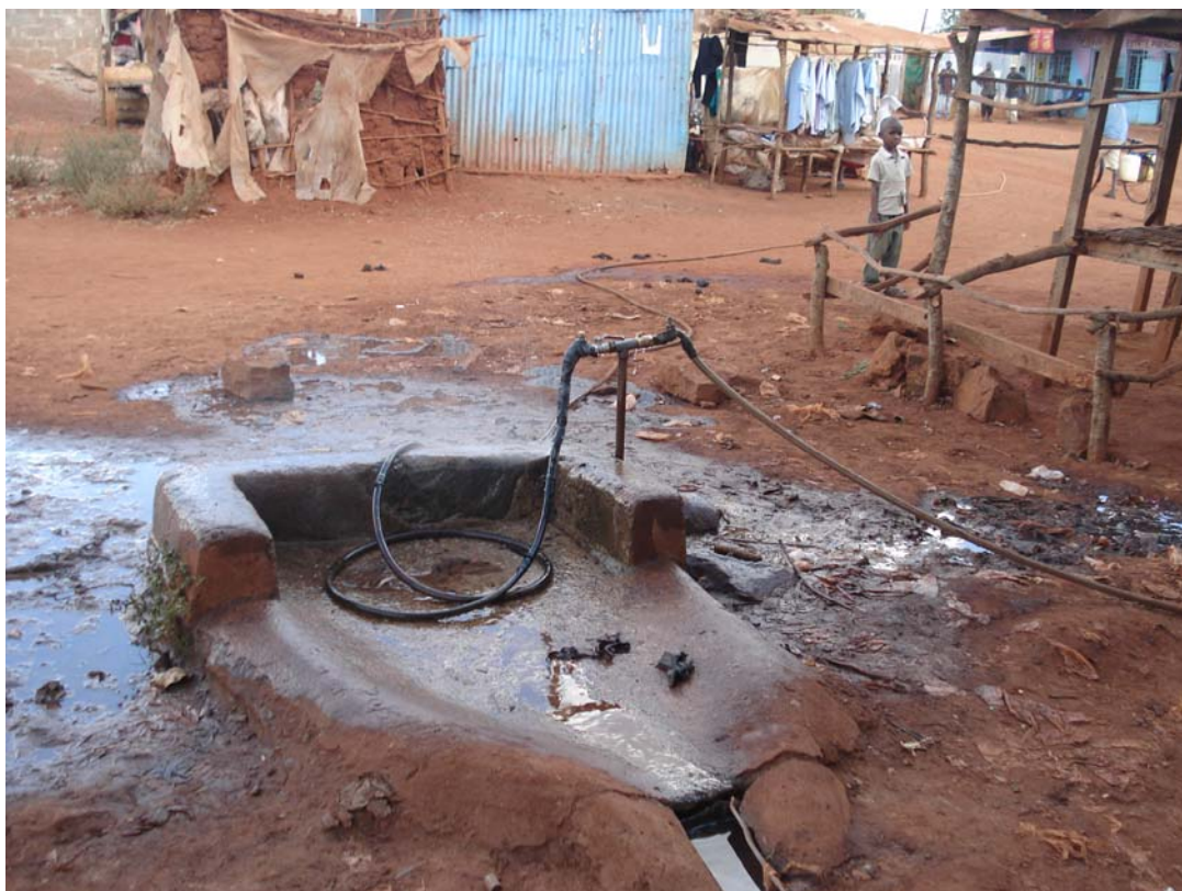
Plate 6: Piped water supply
