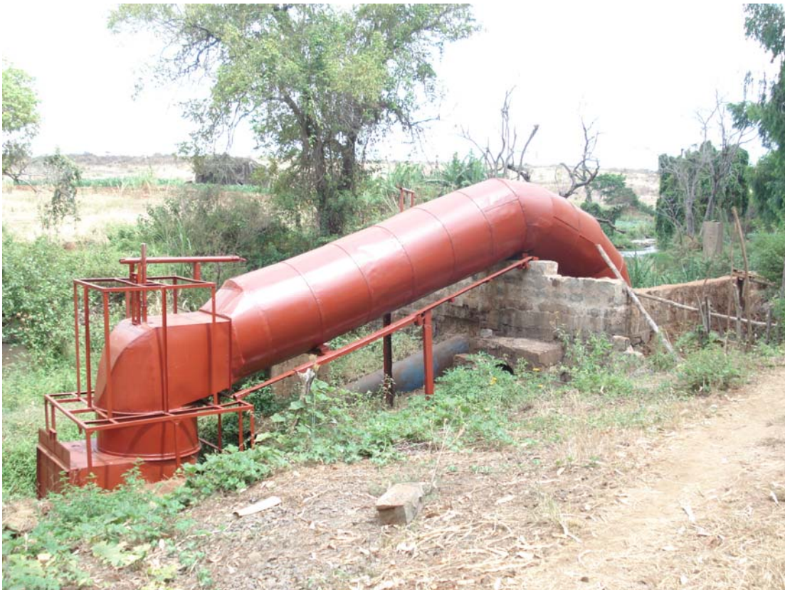
Plate 11: Water abstraction along Rupingazi using installed pump
