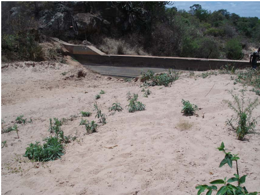
Plate 5: Silted Kigondore concrete dam
