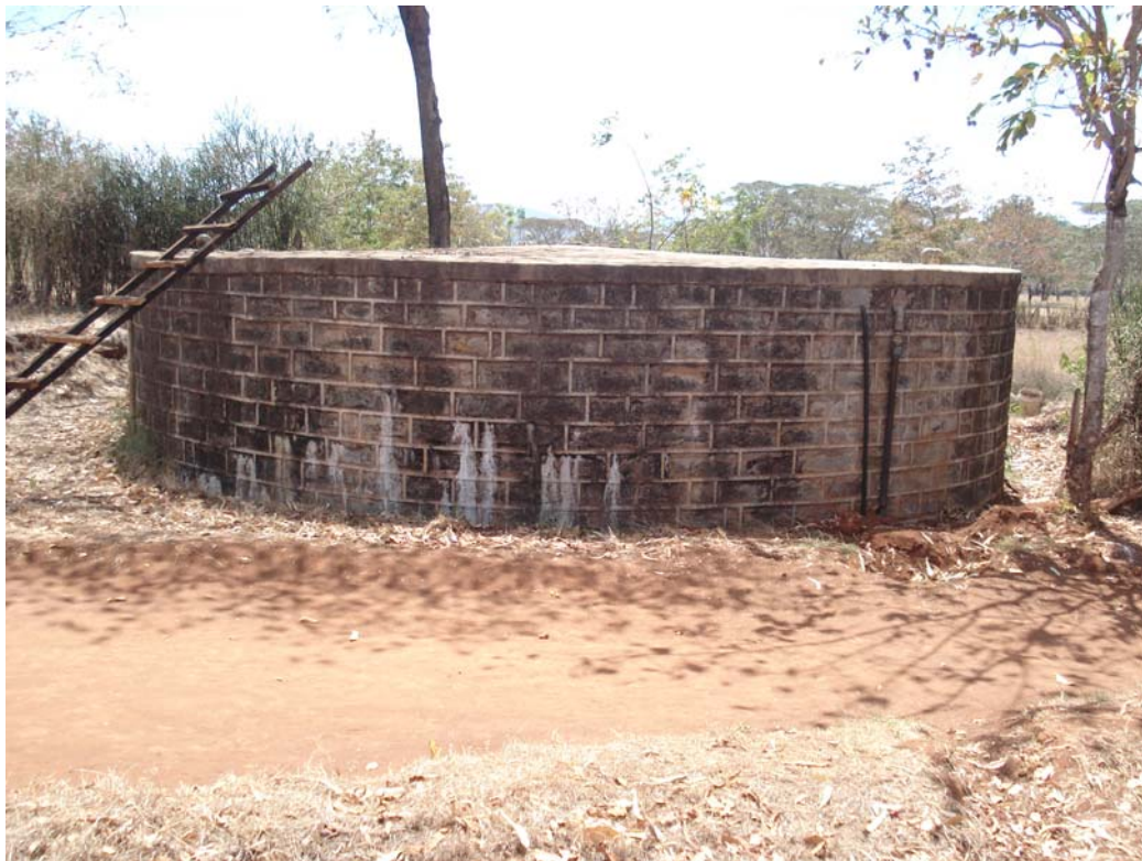
Plate 2: Water supply tank
